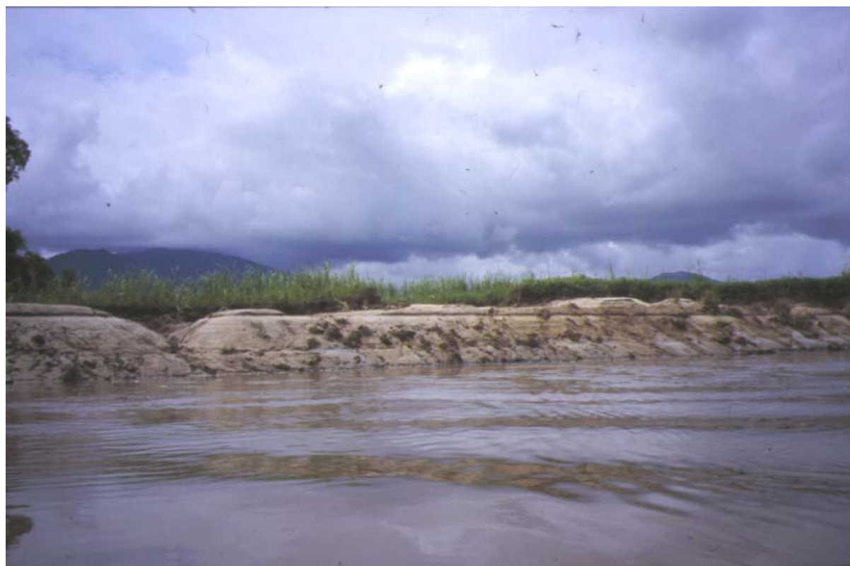
Plate 2. Bank erosion on Thomatis Creek after the 1998/99 floods.
