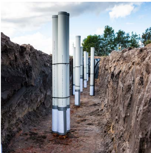
Figure 4.4 Installing a bioreactor wall for a research trial with monitoring piezometers within the wall.
