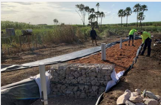
Figure 2 Bioreactor looking from the inlet toward the outlet, showing the rock gabion separating the inlet from the woodchip.
