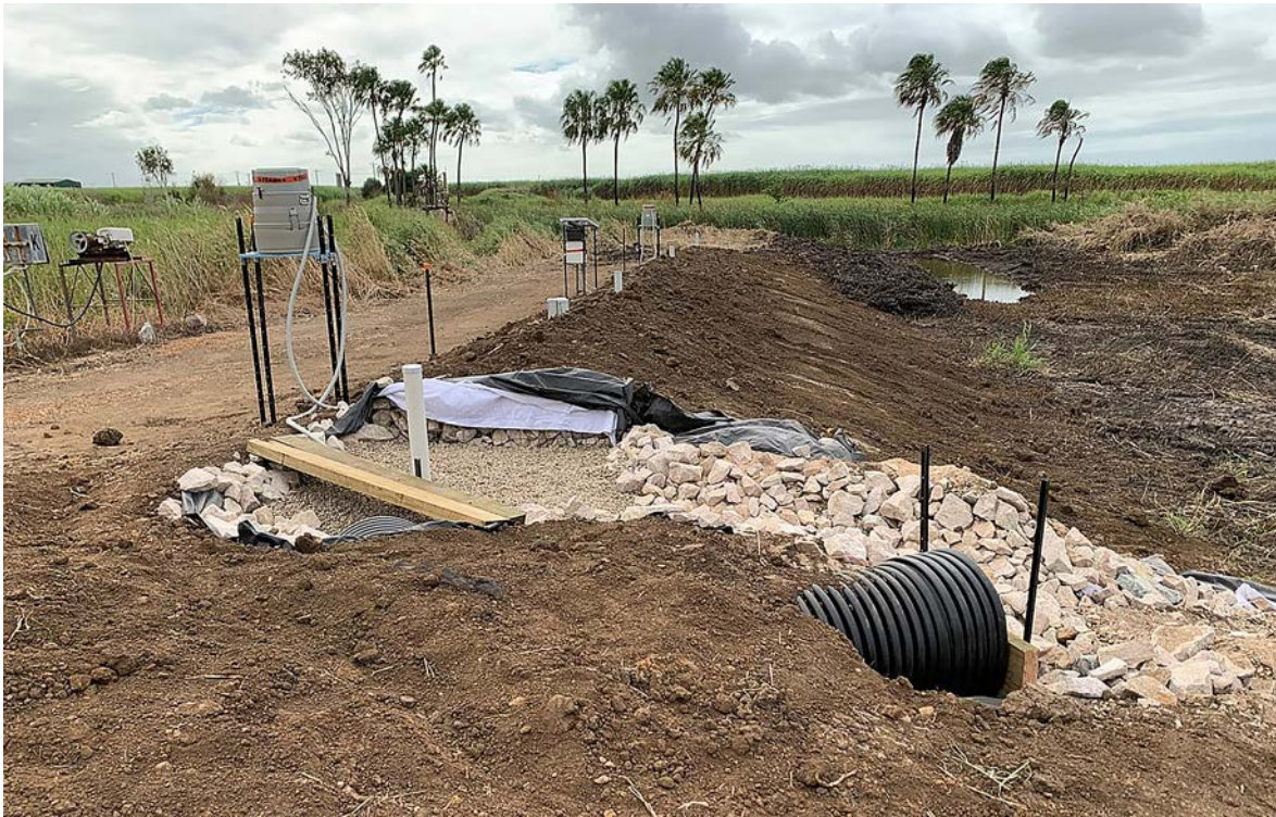
Figure 3.8 Monitoring equipment set up at a research trial site, showing piezometers and automatic samplers.
