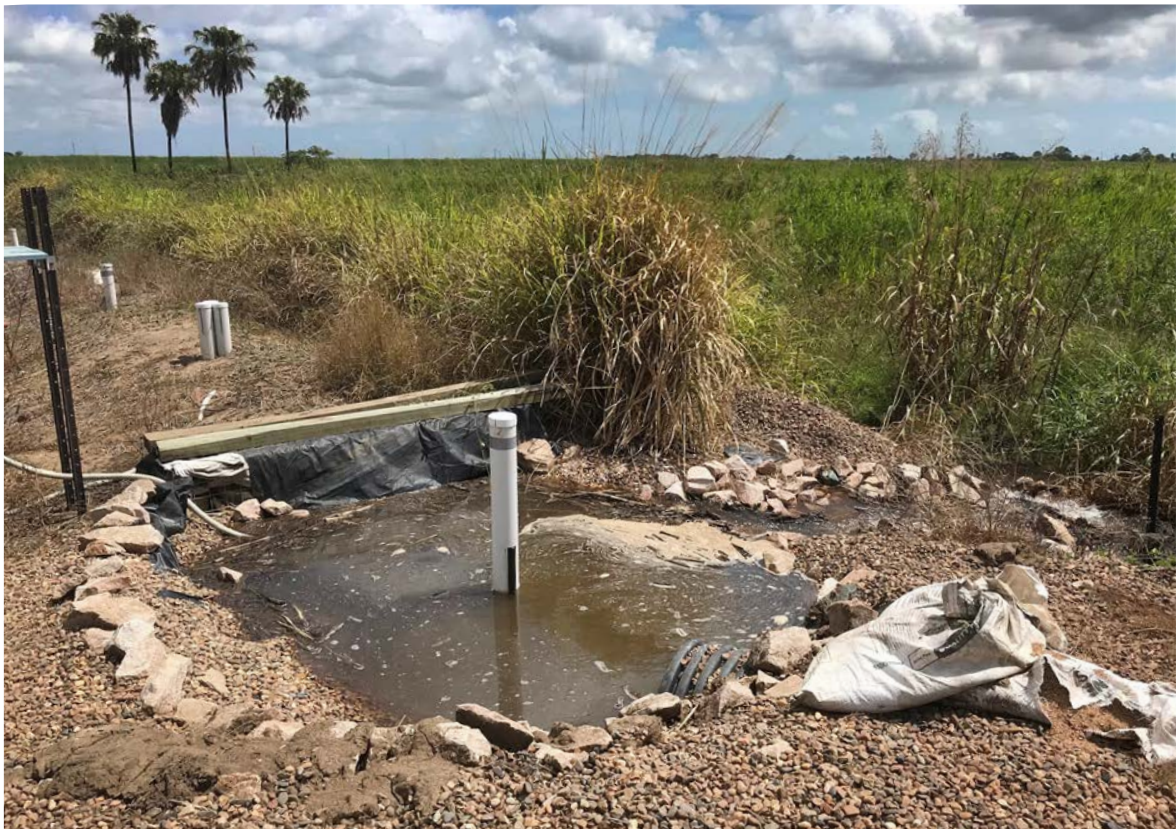
Figure 1.16 Off-line bioreactor bed installed downslope of an irrigated cane block in the Lower Burdekin.
