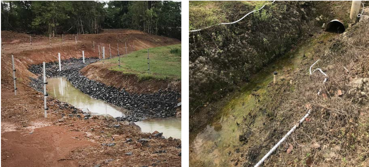
Figure 1.15 Bioreactor beds installed downslope of cane farms in the Wet Tropics region. Photo on left shows in-line bioreactor bed above the floor of the drain. Photo on right shows in-line bioreactor bed below the floor of the drain.
