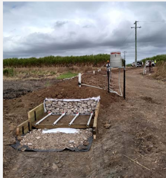
Figure 4 Bioreactor outlet showing four outlet pipes.
