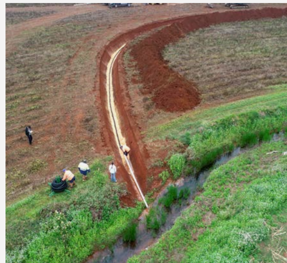
Figure 3 Ag-pipe bioreactor outlet into drainage line. Source: WTMIP
