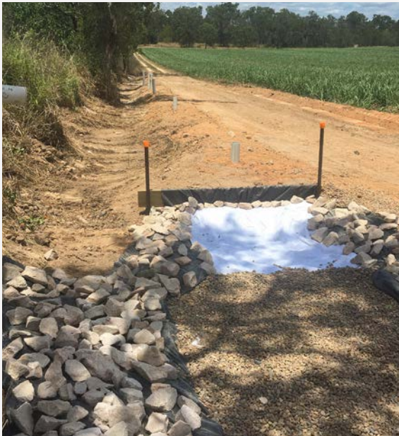
Figure 2 Inlet structure showing washed river gravel and geofabric designed to capture fine sediment.
