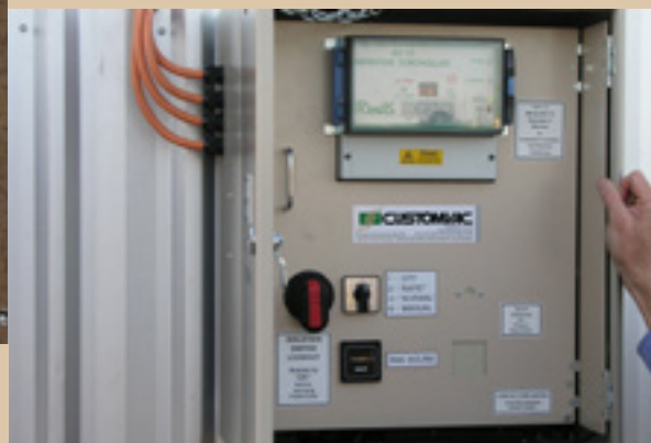
Example of an automatic aeration fan controller used to select optimum ambient temperature and humidity parameters for storage aeration fans
