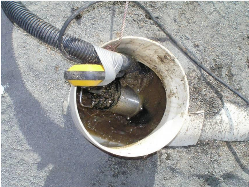
Figure 12: Submersible pump sampling effluent from 225 mm x 225 mm PVC pipeline tee.
