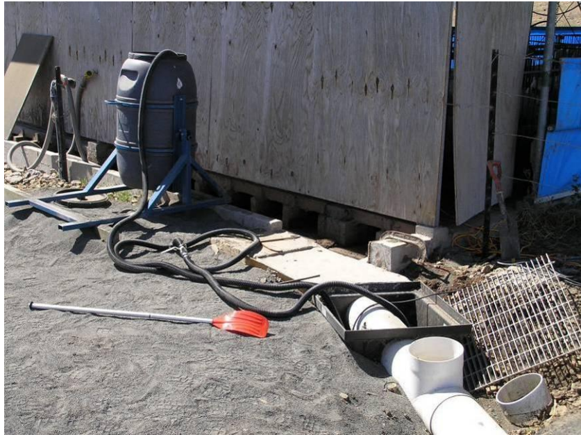
Figure 6: Effluent collection facilities on shed 5, showing the 200 L tipping drum, effluent stirring paddle, 225 mm x 225 mm PVC pipeline tee and polythene sampling sump.
