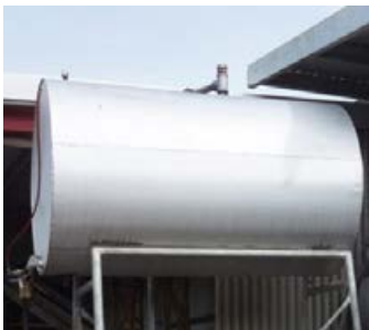
Fuel should only be stored in tanks specifically designed for this purpose.
