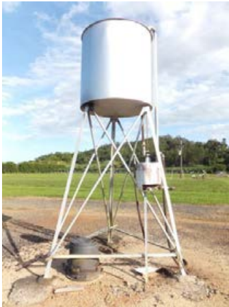
Fuel tanks should be located a safe distance from waterways.
