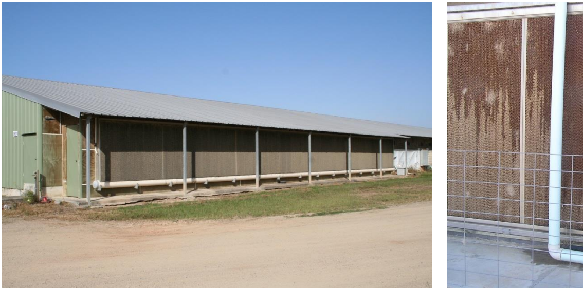
Figure 9. Evaporative cooling cells on a meat chicken shed ( left ) and using water to cool the air entering the shed ( right )
