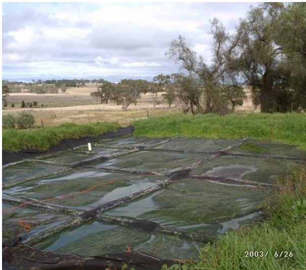
Figure 121: Water ponded on surface of permeable cover 3
