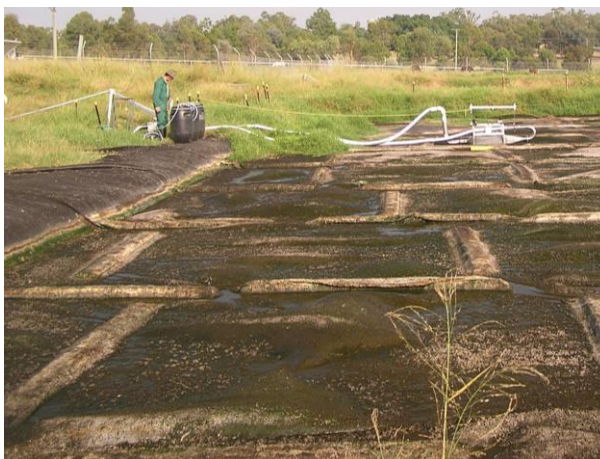
Figure 123: Biomass drying on cover surface to form sludge
