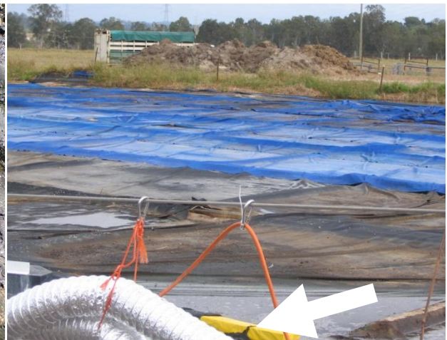
iv) Polypropylene cover 25 months after deployment - continued disintegration of cover not protected from sunlight (June 2005)
