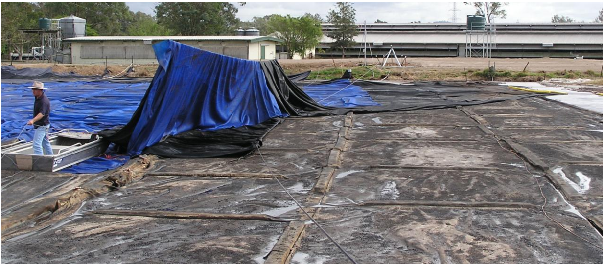
Figure I07: Wind damage to a polyethylene shade cloth cover.
