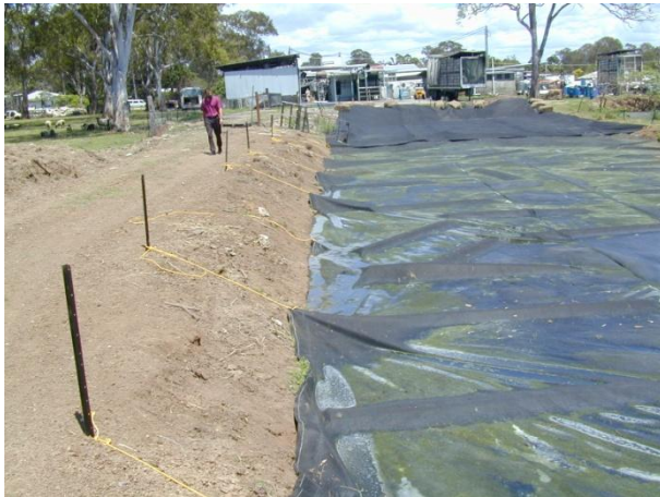
Figure 108: Permeable pond cover immediately after installation – note steep, unstable bank and absence of buoyant material along cover margin
