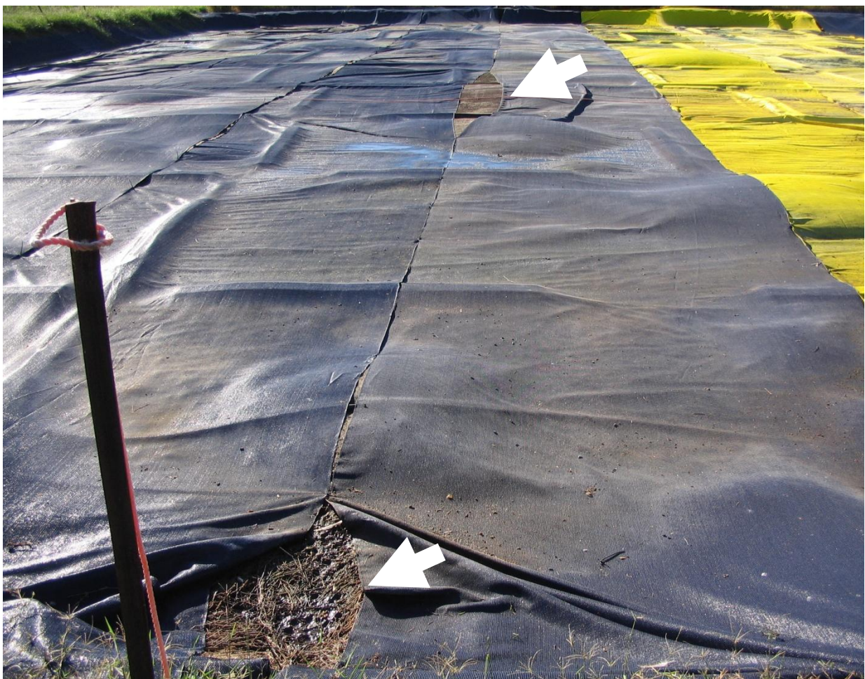
Figure 36: Failure of cable ties used to attach lengths of polyethylene shadecloth following deployment (piggery C)
