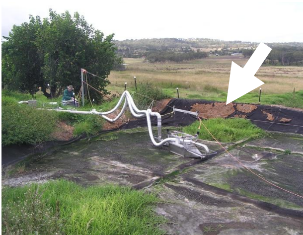
v) Cover after 14 months (April 2004); Note extensive damage (arrow)
