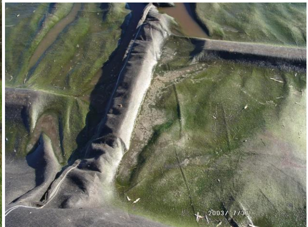
Figure 122: Water ponded on surface of permeable cover 4
