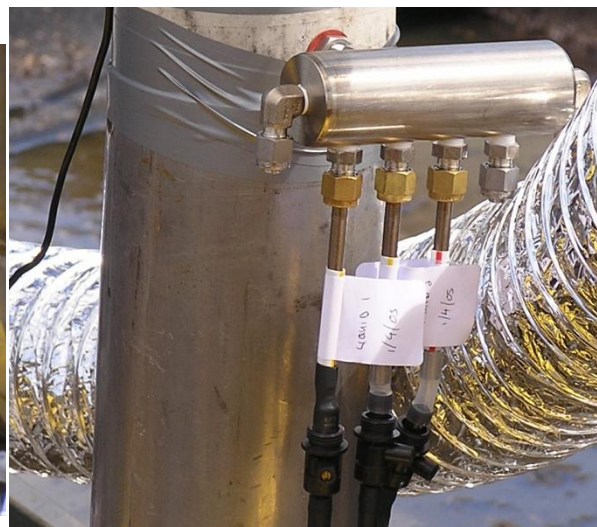
Figure 25: Sample tubes attached to manifold
