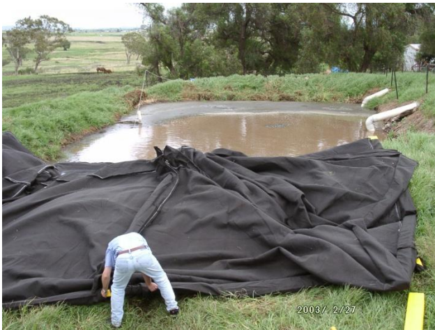
Figure 1: Polypropylene cover ready for deployment
