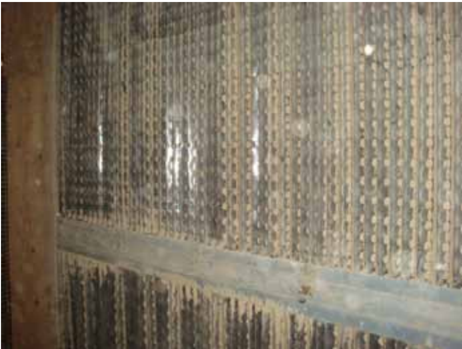
Figure 9 Front face of StuffNix filter. The dust collection tray, covered by a stainless steel flap is visible at the bottom of the filter panel ( Note: filter maintenance had been neglected and required de-dusting )
