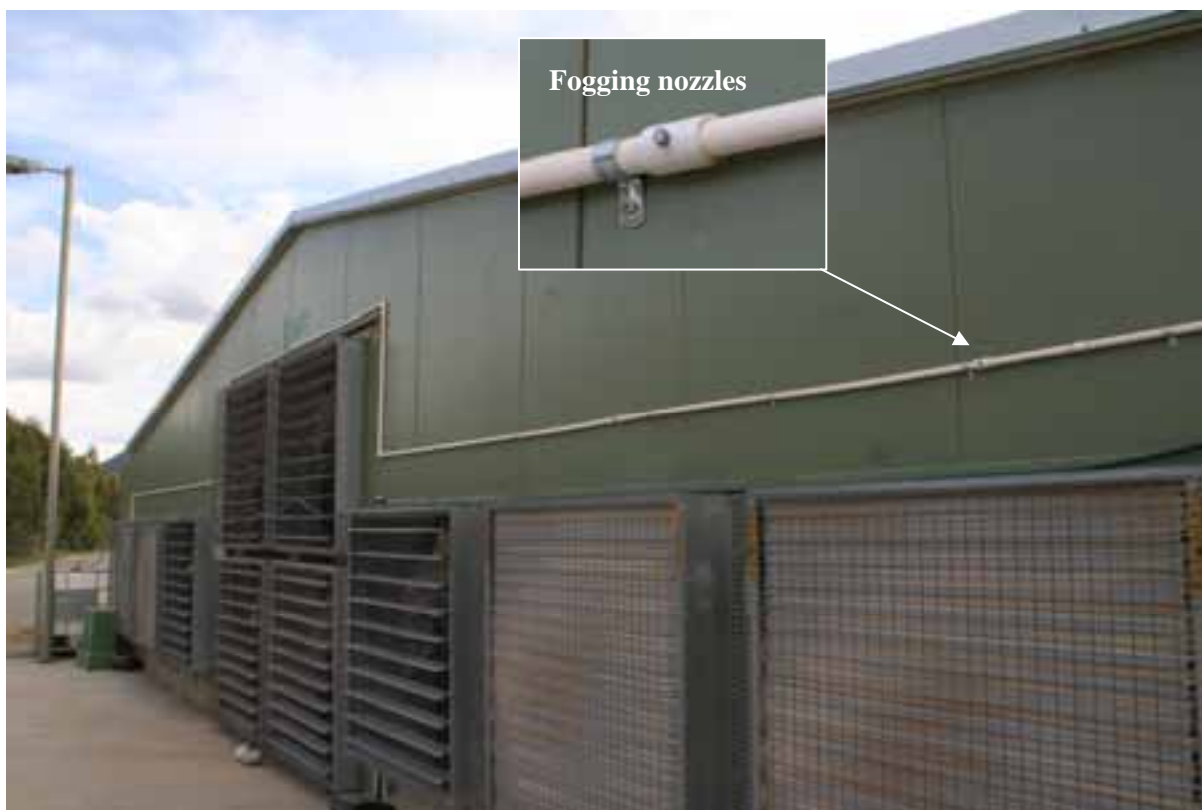
Figure 22 Installation of the Odour Kill system on a SE Queensland broiler farm
