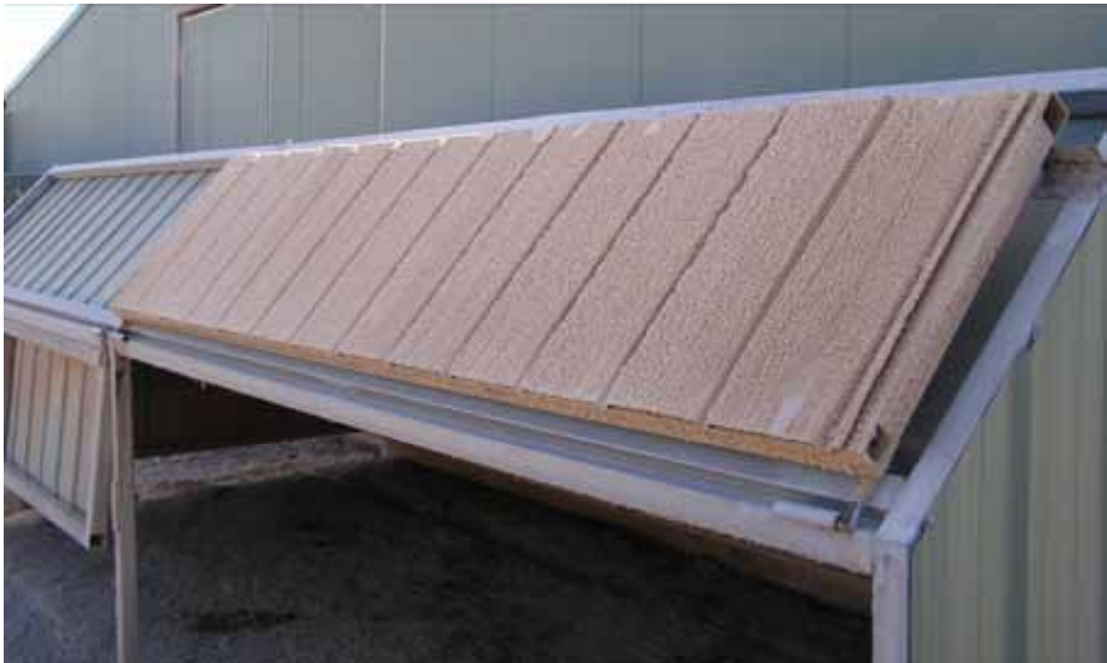
Figure 35 The hood shown in Figure 34 with access flap raised to show visible accumulation of dust
