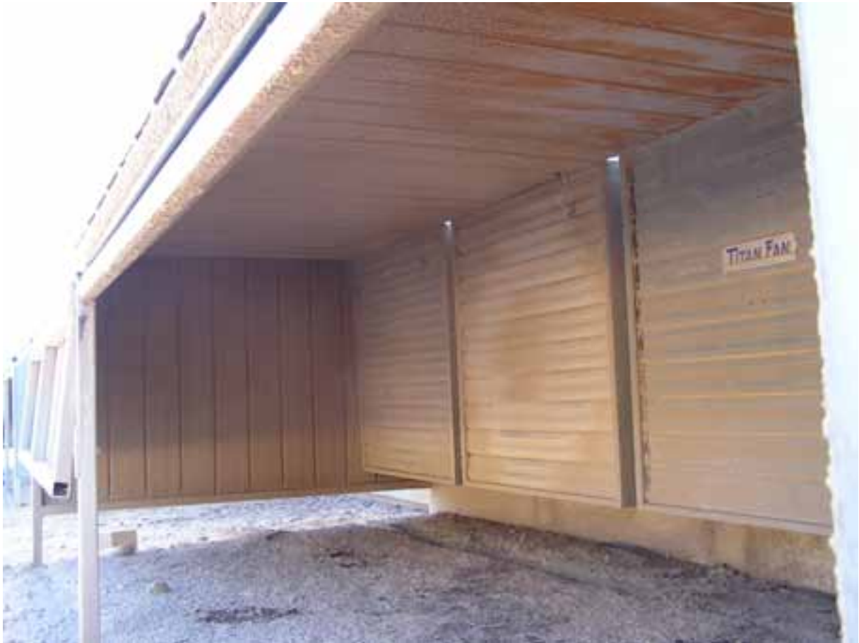
Figure 36 Interior view of the dust hood shown in Figure 34 showing the visible accumulation of dust
