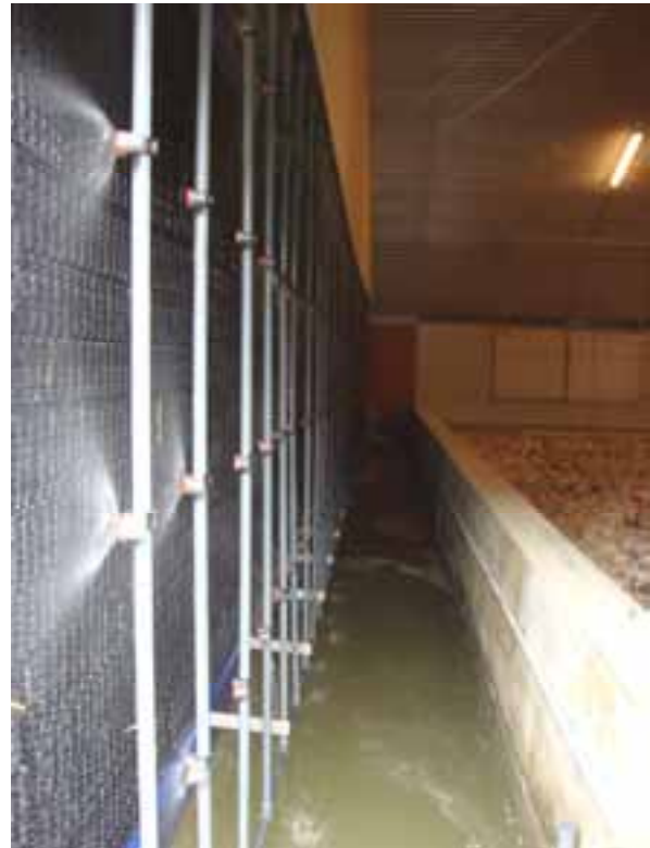
Figure 14 MagixX system installed in a poultry house in Germany - front view of the filter bank showing spray nozzles, proximity to chickens and warm weather ventilation fans on far side wall
