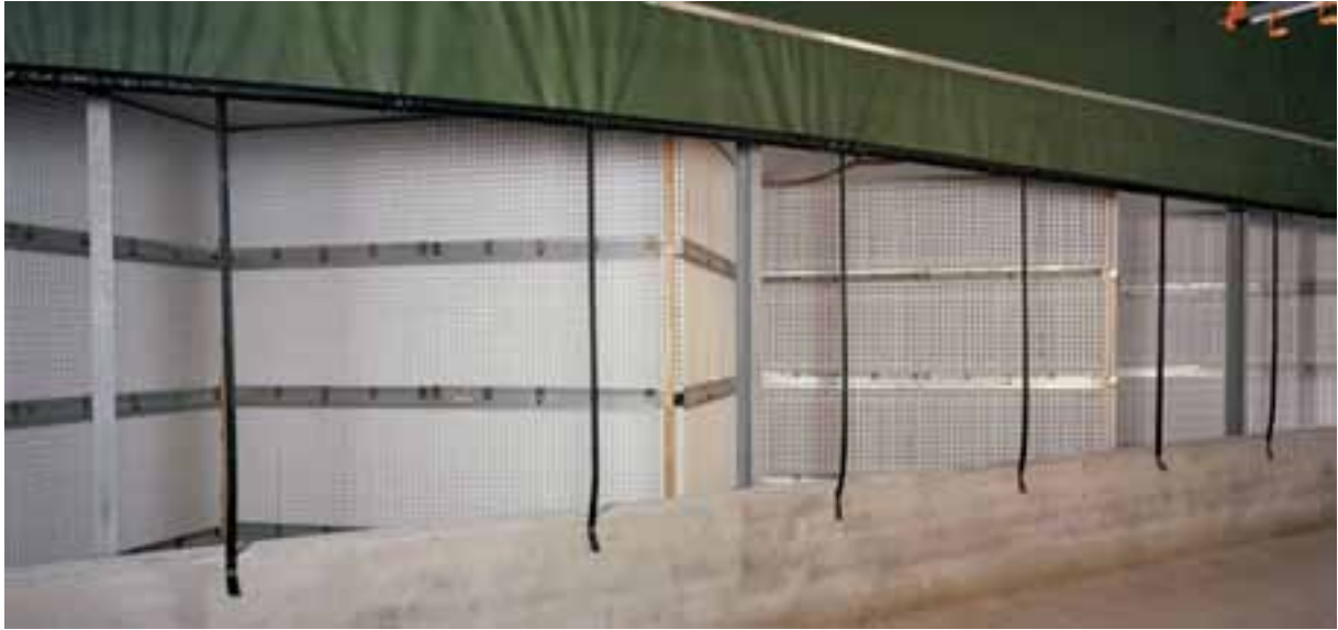
Figure 1 StuffNix filter system installed in a poultry shed (original, superseded, paper filter panels were used in this installation, source: http://www.bigdutchman.de/bd_images/fotoseiten/Stuffnix.jpg )
