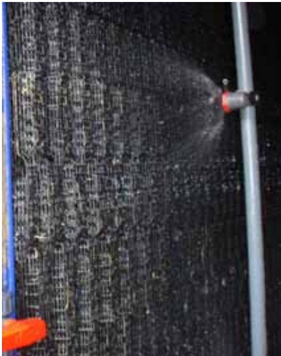
Figure 17 MagixX: close-up image of the filter bed structure
