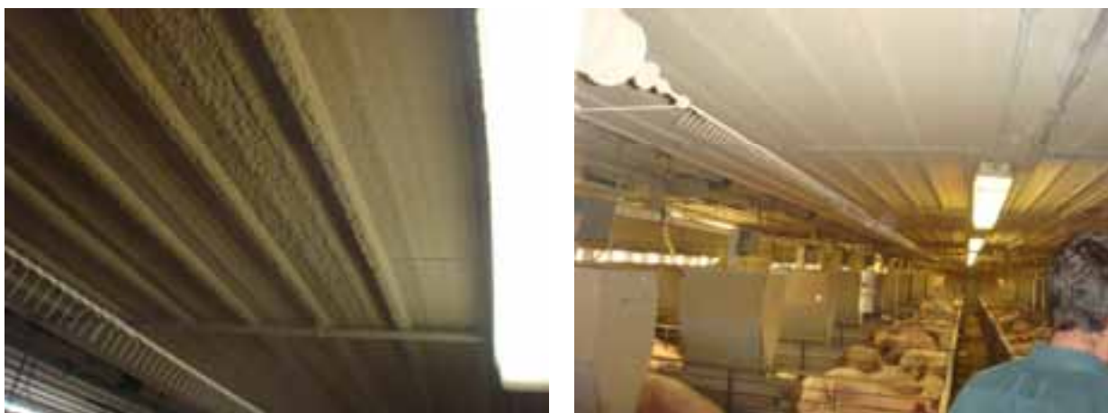
Figure 26 Accumulation of dust on the ceiling directly above the EPI system (left and right)
