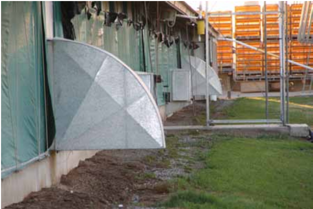
Figure 33 Hoods placed over 915 mm (36”) fans to direct dust and feathers downward
