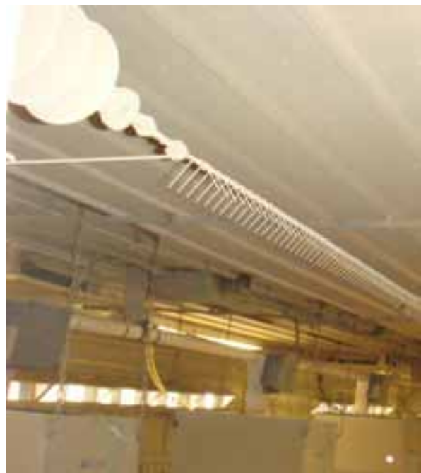
Figure 25 Stainless steel ionization wires with sharp pointed electrodes (insulator on the top left side of photo)
