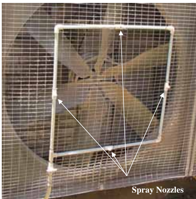
Figure 23 OEC water sprays mounted on the outside of a ventilation fan
