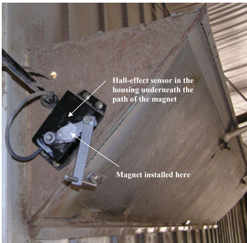
Figure 7 Mini-vent position sensor following installation of a Hall-effect sensor and magnet
