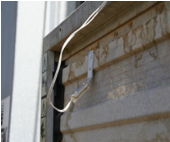
Figure 4 Mercury tilt switch with fan turned off (shutters closed, switch closed)
