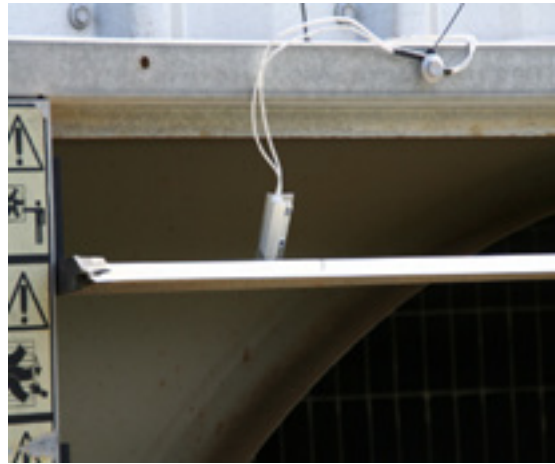
Figure 5 Mercury tilt switch with fan turned on (shutters open, switch open)
