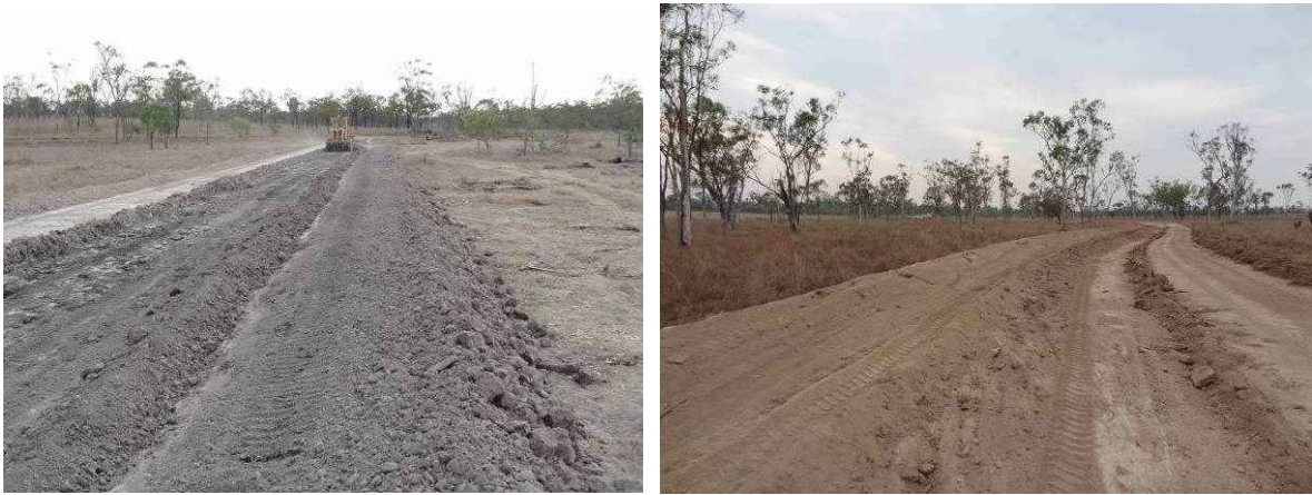
Image 11. L. Grader constructing creek over-flow diversion bank; and R. Contour bank to direct hillside water off experiment site at Spyglass (Oct. 2011).
