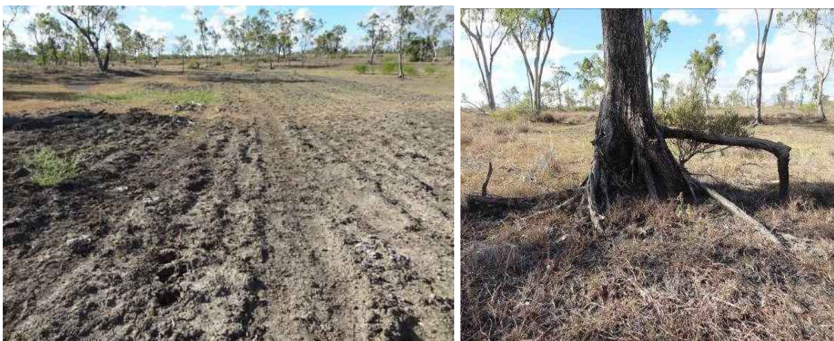
Figure 5. Gypsum strip on clay soil, no pasture establishment, in River paddock south of double dam (L) and depth of eroded surface at northern end of the hollow (R). Note: gypsum truck tracks are still evident after a full summer (19/03/14).
