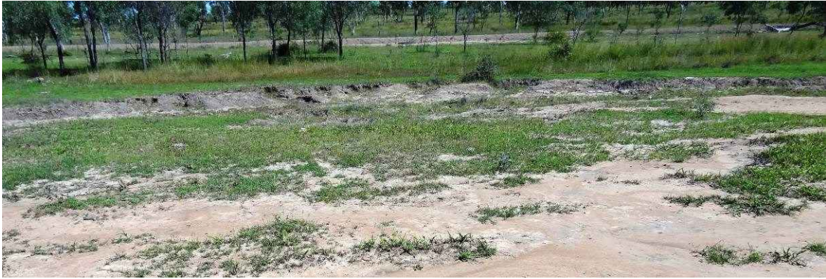
Image 14. Eroded edge (50 cm deep) along south side of Spyglass experiment site with upper-slope contour bank above tree line controlling hillside water movements (April 2013).
