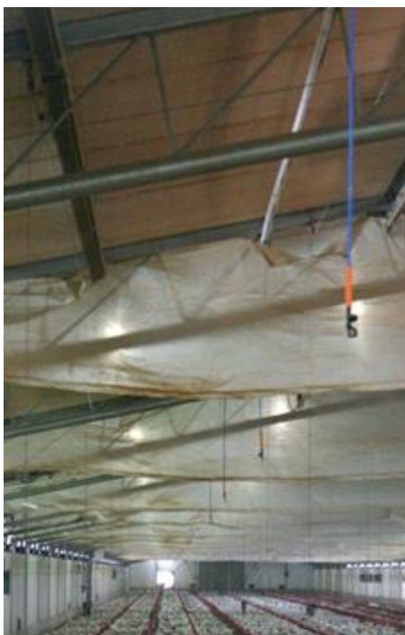
Figure 1. Sprinklers suspended from the ceiling in a meat chicken shed
