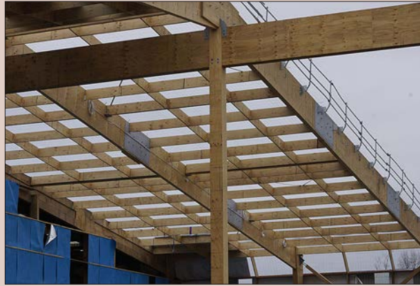
Figure 2.8. Laminated veneer lumber roof structure. Photo: Engineered Wood Product Association of Australasia.
