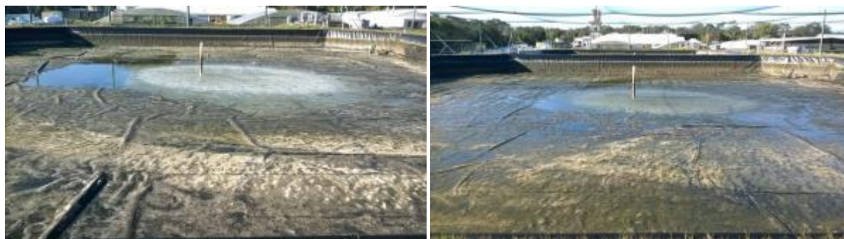
Figure 10 Pictures of recently drained ponds G1 (left) and G2 (right) showing accumulated piles of sludge.
