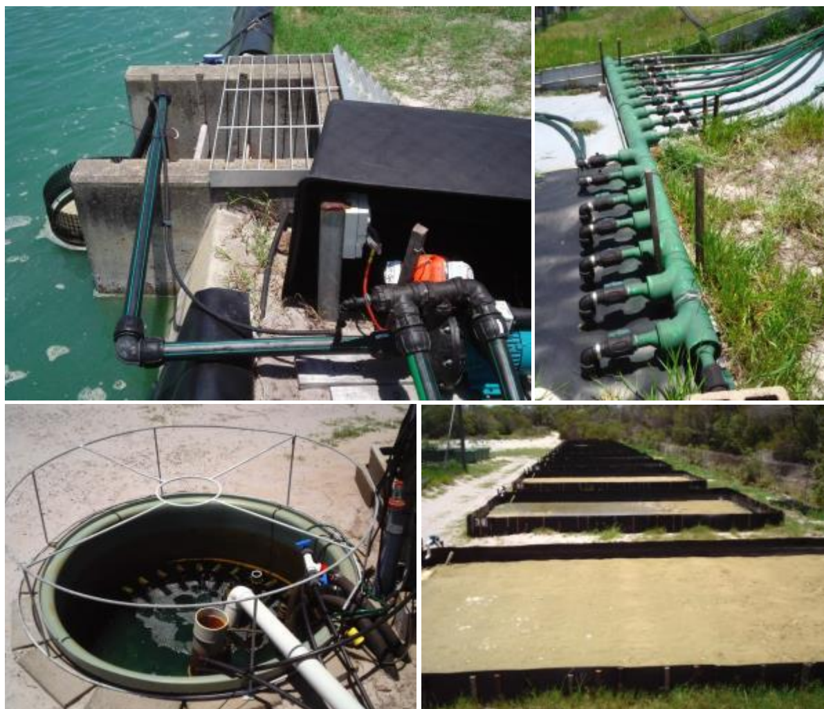
Figure 2 Construction of the PASF recirculation system at BIRC showing one of the pond water supply pumps (top left), the pond water mixing manifold (top right), the filtered-water collection sump (bottom left) and the completed PASF beds (bottom right).
