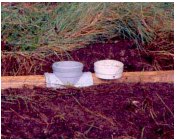
Figure 5: Installing a termite aggregation station with the plastic T piece and timber.
