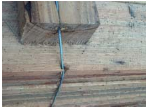
Figure 5.14. Undesirable: No corner protectors
