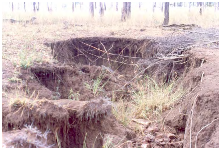
Figure 10.7 Gully erosion that will occur on our poplar box country if the surface A horizon is breached by erosion or deep surface disturbance, e.g. by roads.
