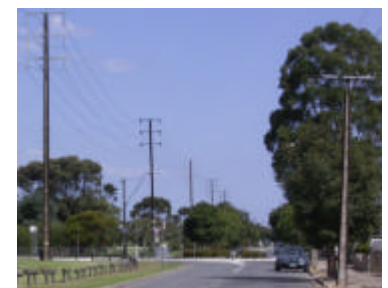
Figure 2 Typical Stobie poles in-service
