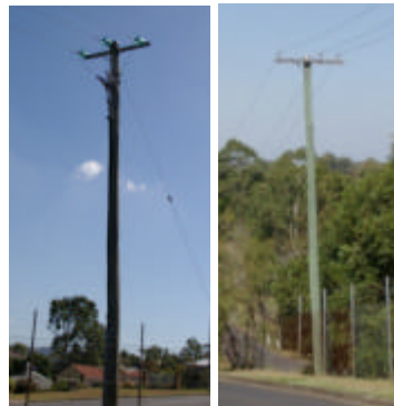
Figure 1 Typical timber distribution poles in-service
