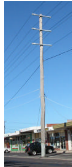
Figure 28 Rebuttet pole in-service for 20 years (courtesy Mr Doug Cowey, Pole Rebutters Australia)
