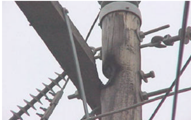
Figure 15 Damage caused by pole-top fire (courtesy Mr Dennis Clancy, PowerCor Vic.)
