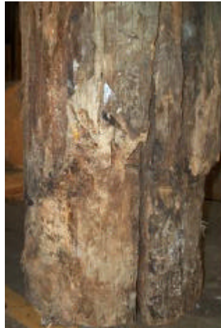
Figure 40 Soft rot around ground-line in decommissioned treated hardwood pole
