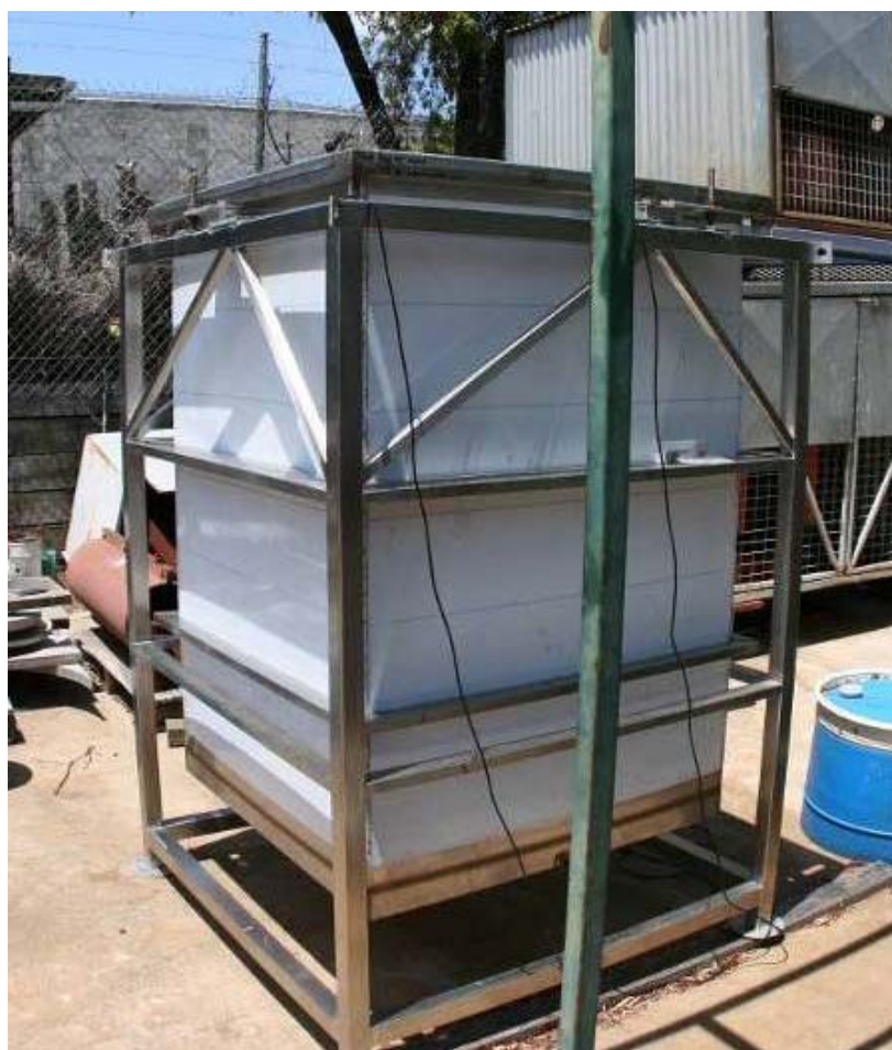
Figure 42. Lysimeter during construction showing the inner box inside the outer box frame.
