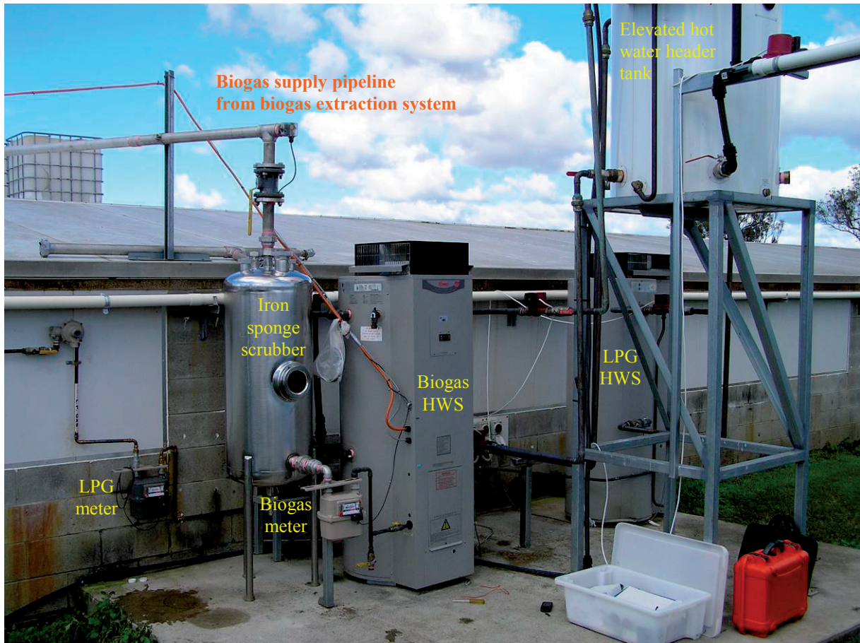
Figure 3. Biogas and LPG water heating systems, biogas scrubber and elevated hot water header tank.
