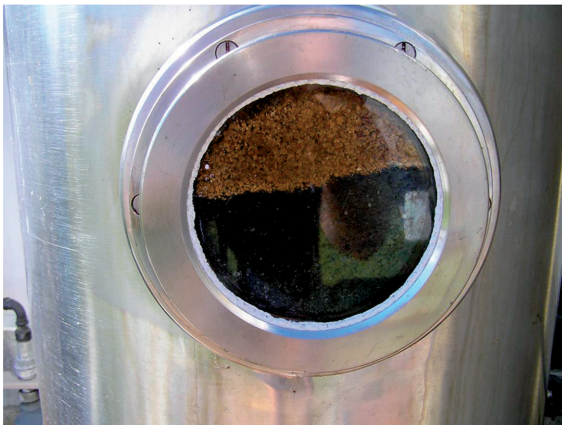
Figure 17. Viewing porthole in the biogas scrubber following the addition of the third drum of SULFA-BIND® showing the black colour of the exhausted medium in contrast to the orange coloured fresh medium.
