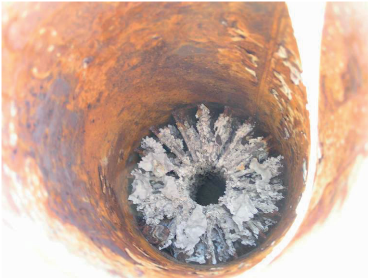
Figure 5. Flaky sulphurous deposit in the baffles of the biogas hot water system flue.
