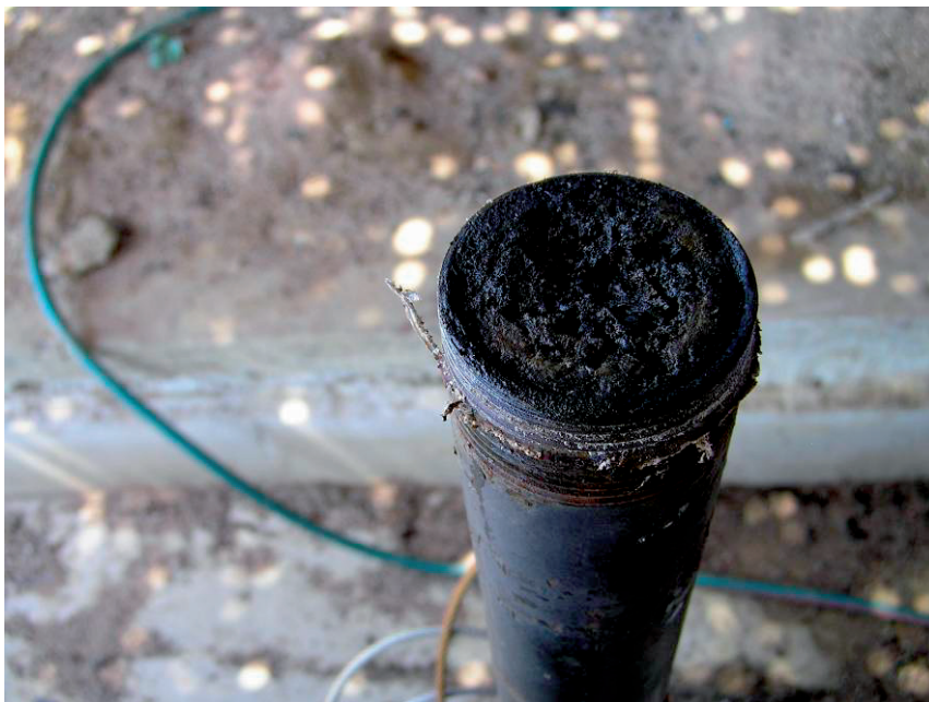
Figure 10. Hard, carbon-rich deposit which had built up on the upper side of the ball valve installed on the stem of the flare, blocking biogas flow.
