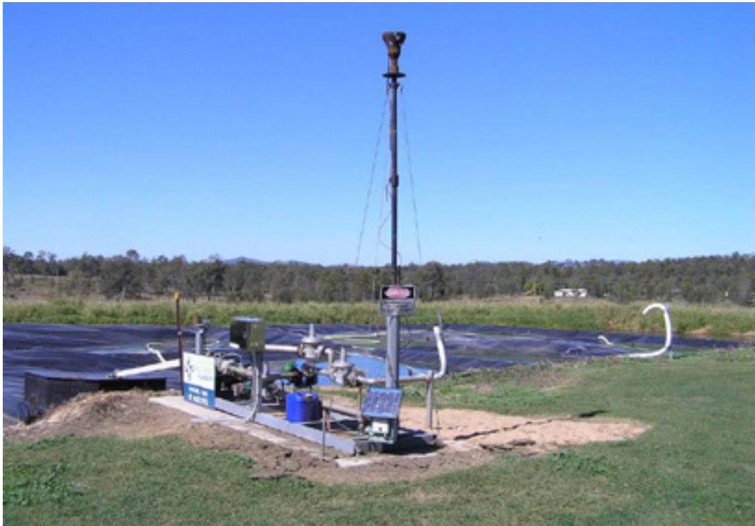
Figure 4. Biogas extraction system installed adjacent to the north-western corner of the primary effluent pond.
