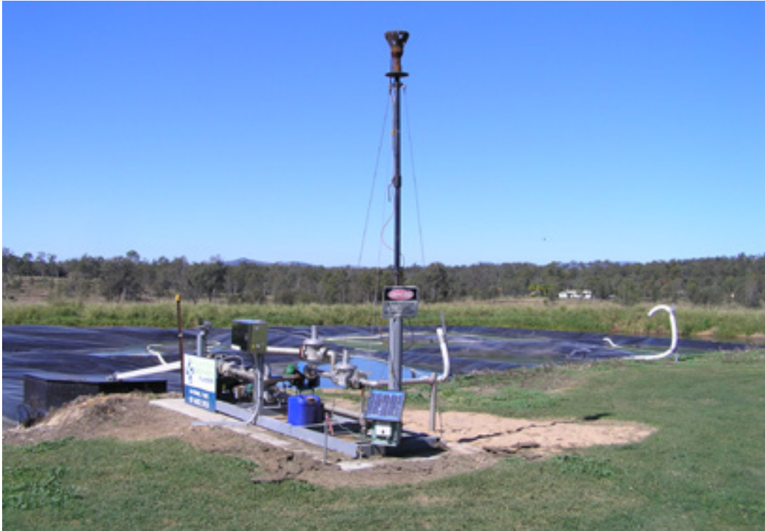
Figure 27. Biogas extraction system installed adjacent to the north-western corner of the primary effluent pond.
