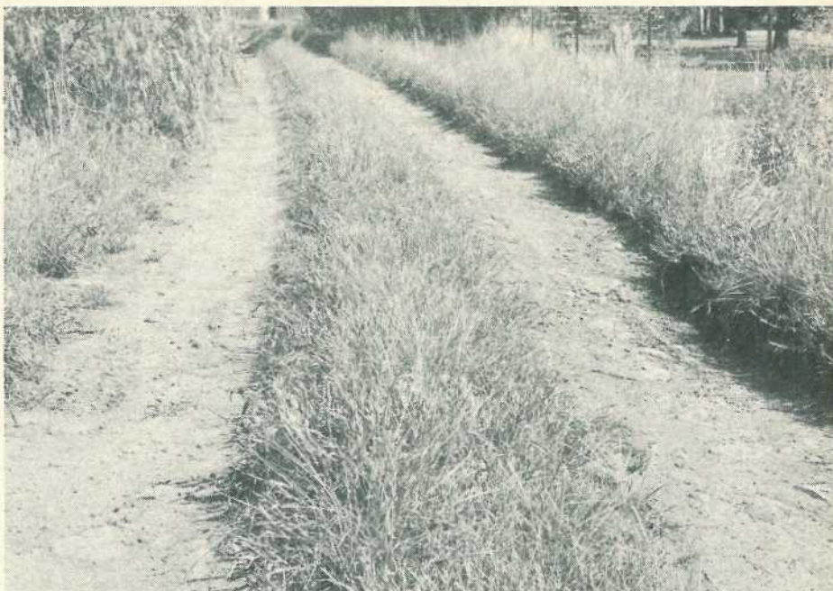
An example of poor construction and lack of drainage.
