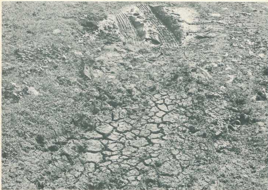
One of the problems associated with poor planning—lack of drainage.
