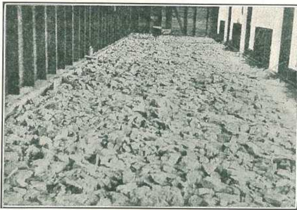
Fig. 2.—Rock foundation for cement floor. This prevents the moisture from coming up from the soil below. A floor on such a foundation should be dry.
