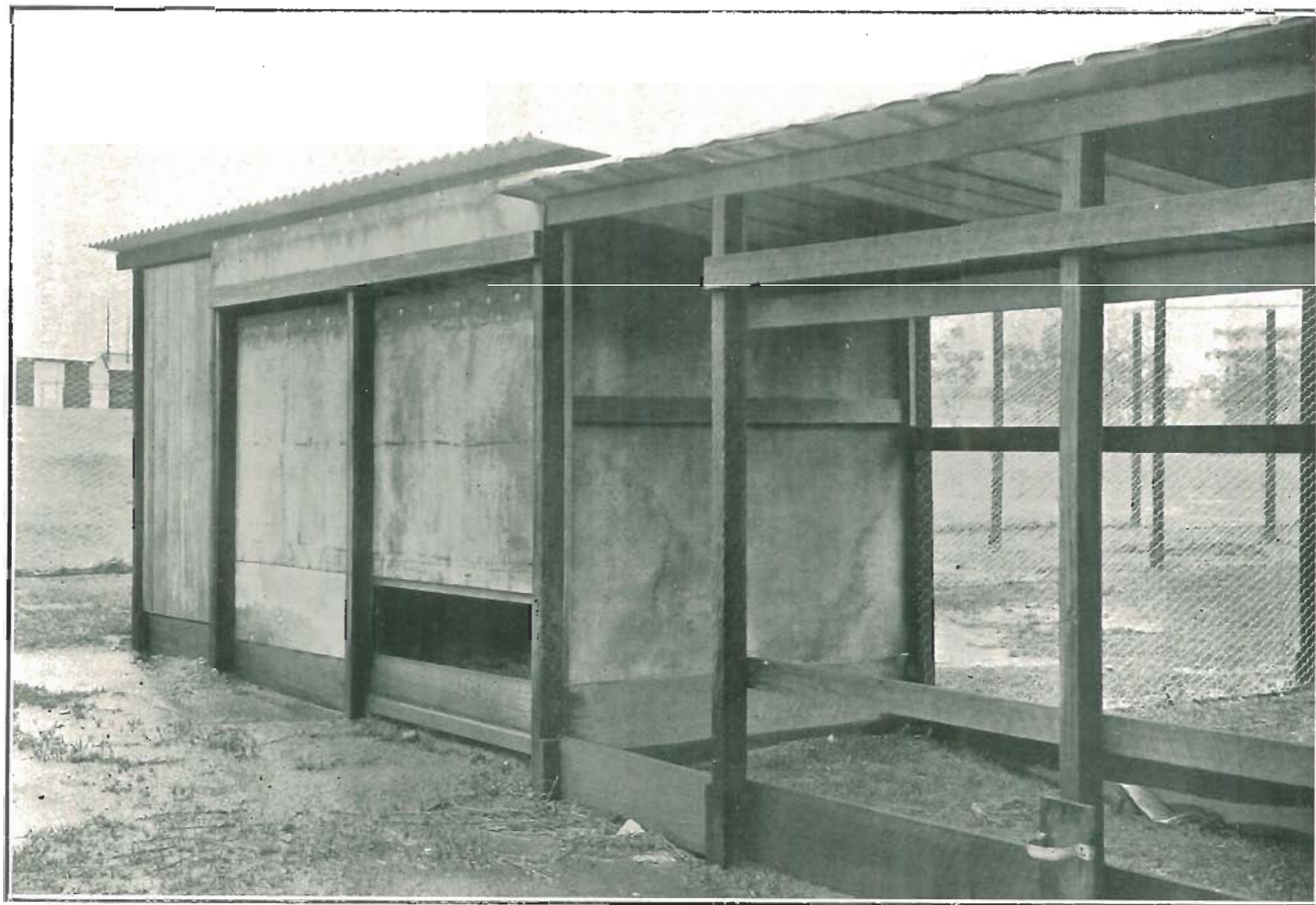
PLATE 25.—BACK VIEW, SHOWING A COMPLETED HOUSE AND FRAMING WALLED WITH ROOFING FELT.
