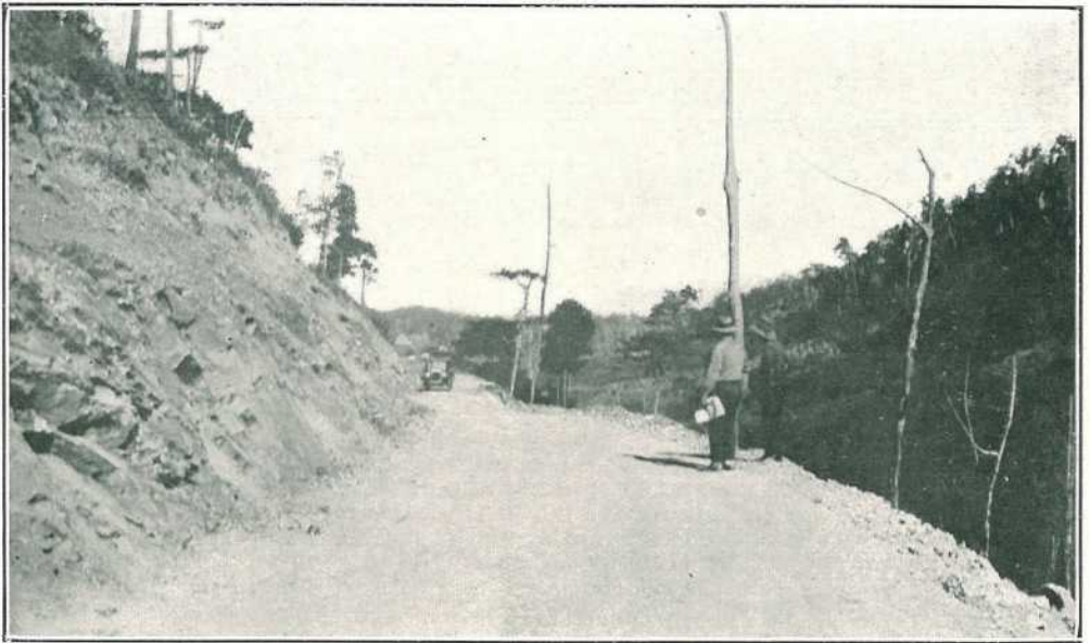
PLATE 11.—PIONEER SHIRE. Mount Ossa-Kungurri Road, which will serve recent settlement in sugar-growing country.
