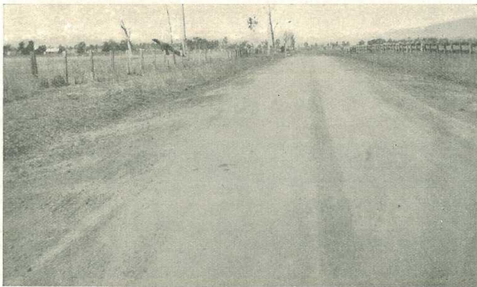
PLATE 160.—TARAMPA SHIRE—LOCKYER-DARLING DOWNS HIGHWAY (BRISBANE-TOOWOOMBA SECTION). A further section of road effectively treated by the heat process.
