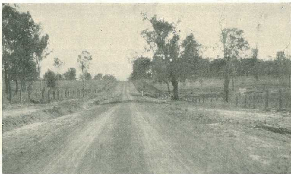
PLATE 159.—ROSEWOOD SHIRE—WALLOON-HAIGSLEA ROAD. A section completed by the use of the Irvine Heat Treatment process.
