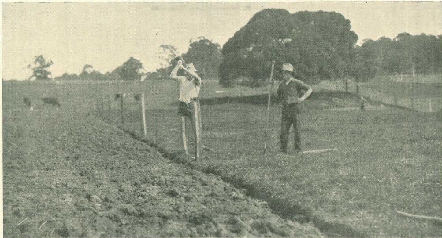
PLATE 114.—WIELDING THE MAUL. A temporary stake fence to enclose a fine sward of Italian rye grass (right) on St. Lucia, in course of erection.
