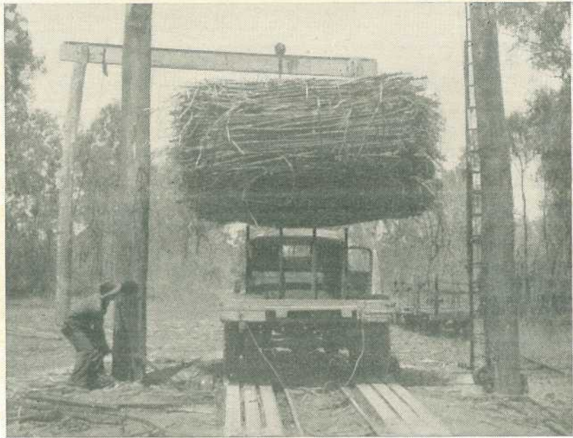
Plate 68. APPLYING THE BRAKE AFTER THE LOAD IS RAISED FROM THE MOTOR TRUCK.
