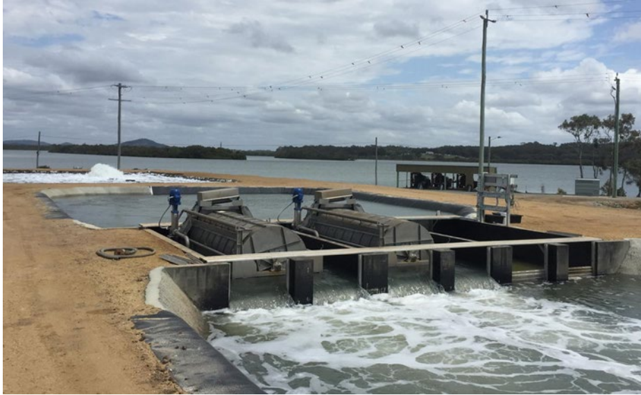
Figure 5. Rotating drum filters in original configuration as used in Season 1. Note the small pond, in the background (sampling location #1) receiving raw water pumped from the Logan River, and filtered water flowing into the farm distribution channel in the foreground.
