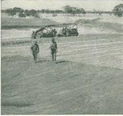
PLATE 1.—Water is the key of life for man and stock in the sheep country. Modern equipment puts down an excavated tank on a western Queensland sheep run.
