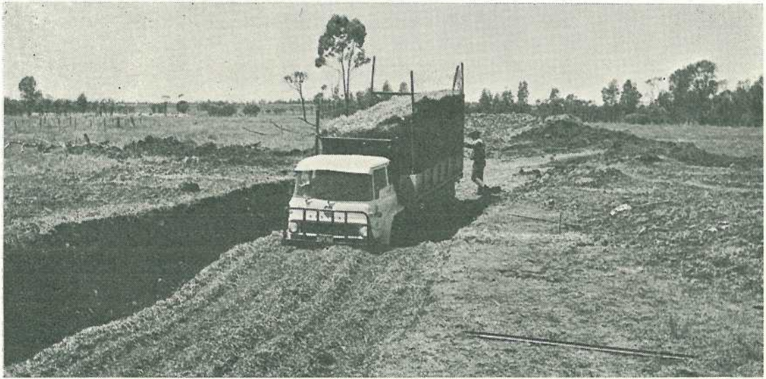
Filling a pit is made easier if the truck can drive through.
