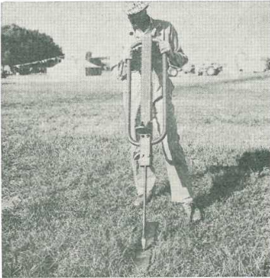
Photo. 26 A Plesse Pylola is used for putting down pilot holes for posts. The diamond point is rammed down in post driver fashion. Two bolts near the bottom of the handles act as stops so that when bumping the bar upwards out of the hole, the bolts contact the head of the bar which slides inside the hollow section. The ledge can be used for driving running posts though close fitting drivers allow better control of the post. (Paragraph 114).
