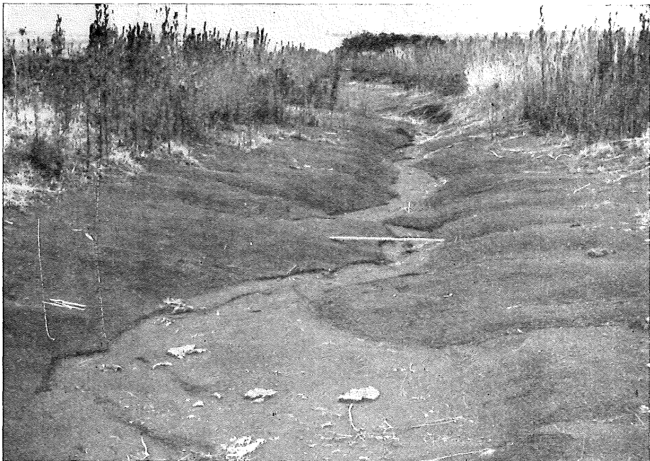
Fig. 10.—Grass was not planted in this scrub soil waterway nor has self-sown grass appeared. The centre gully is up to 2½ ft deep. Waterway 8 in Table 2.
