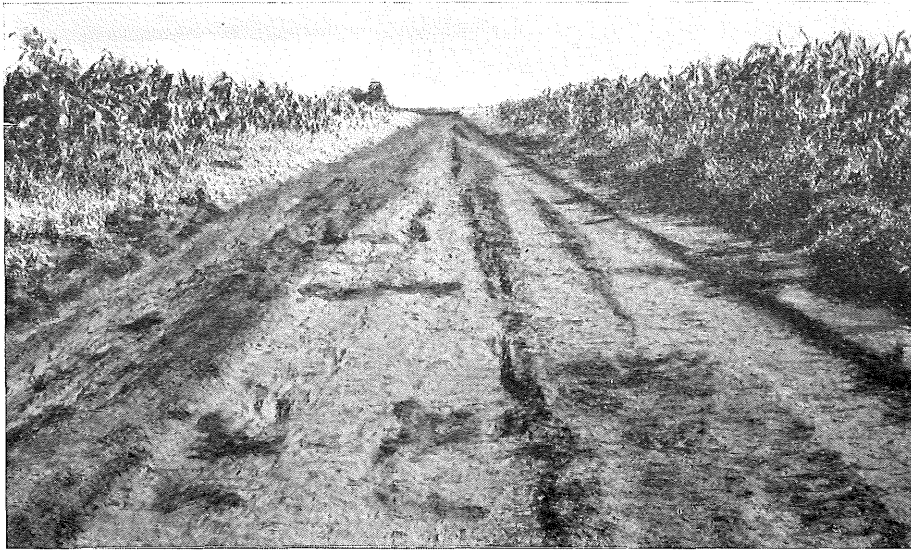
Fig. 3.—Same waterway as Fig. 1 on 17.ii.1956 after a fifth flow in which the waterway flowed at full capacity at a calculated average velocity of 11 ft./sec. The waterway floor is quite bare and perennial grasses planted on the banks have made little growth.
