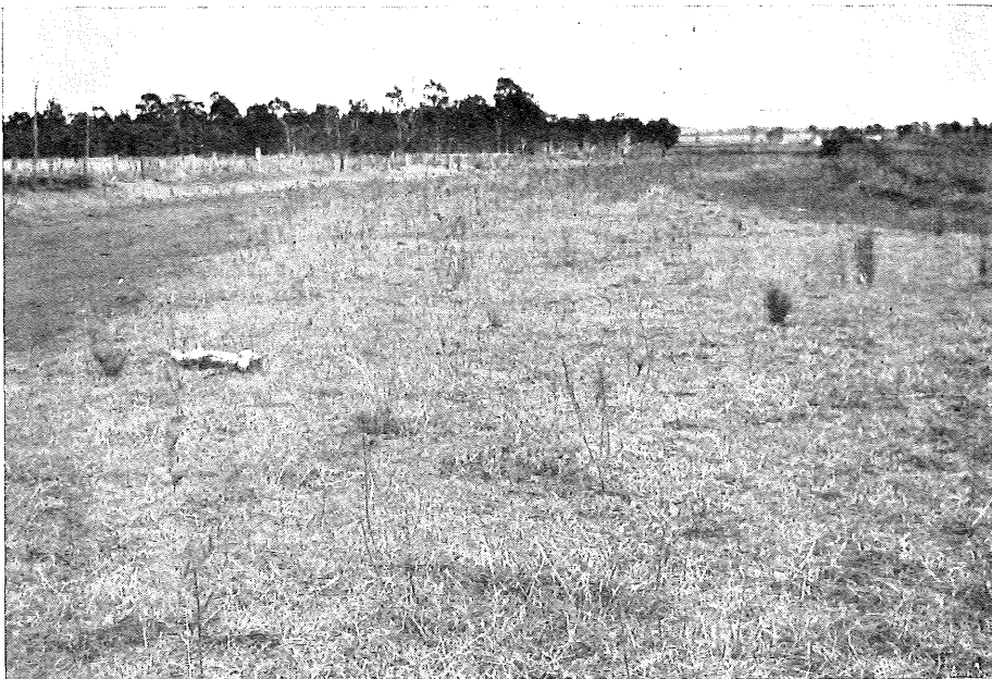
Fig. 12.—A wide forest soil waterway catering for run-off from a 1,500 ac. catchment. Excavation is confined to a strip 25 ft wide on each "side." Waterway 13 in Table 3.
