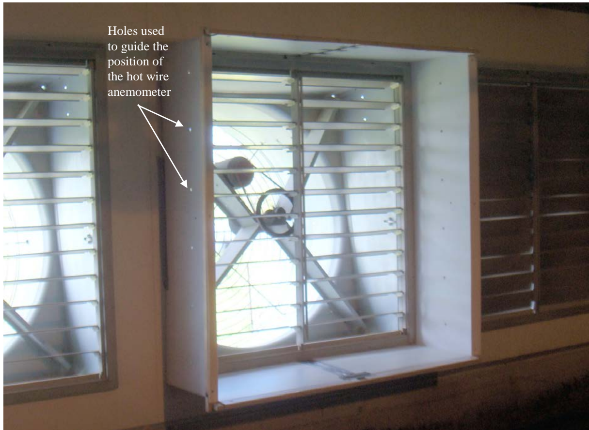
Figure 5. Picture of a temporary cowling used to define a square sampling plane on the inlet side of the fan. Note the holes drilled in the cowling to positively locate the horizontal sampling traverses
