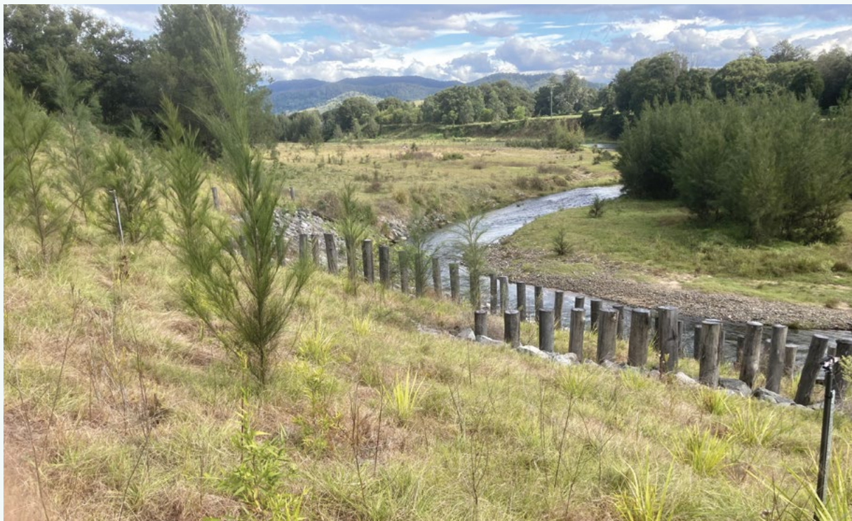
Figure 33. A pile field, riprap, fencing and planting project established in 2020 on the Kenilworth reach of the Mary River. This project had dual objectives of stabilising a streambank to protect local assets and to reduce the delivery of sediment downstream. The project was co-funded, with Reef Trust funding revegetation of this site and of large extents of the reach either side of the engineering works.
