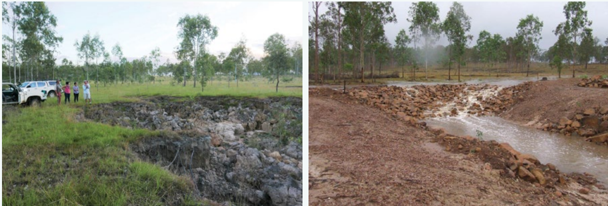
Figure 22. A rock chute installation in the Mary catchment. Left: Before construction in April 2016. The gully had an extensive catchment area, and the gully head was advancing across a small floodplain with highly dispersive sub-soil. Right: After the first major rainfall event in March 2019 (note the same clump of trees on the left of both images). The first runoff event had a 2-year flow recurrence interval, following 126 mm of rain over 3 days including 83 mm within a few hours. Total cost of the rock chute was $55,000, plus the land manager provided approximately $100,000 in-kind contribution primarily in the cartage of rock material from a quarry on the property. The estimated direct cost per tonne of sediment saved was $340/t/year fine sediment reduction at the river mouth, or $1,153/t/year including the in-kind costs.
