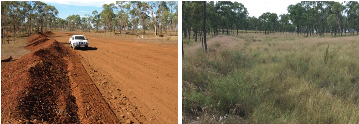
Figure 17. Diversion bank built to divert an 8 ha catchment away from a large gully, which was reshaped and revegetated in the upper Burdekin catchment. Left: Newly constructed diversion bank with topsoil (light brown soil) replaced across the channel area in May 2016. Right: Same location in April 2019. Livestock were excluded from the area for 3 years to assist revegetation.
