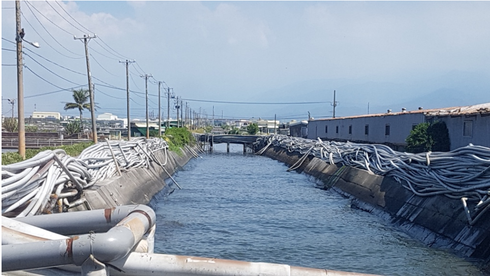
Figure 11: Crazy network of water supply pipes in Ping Tung County
