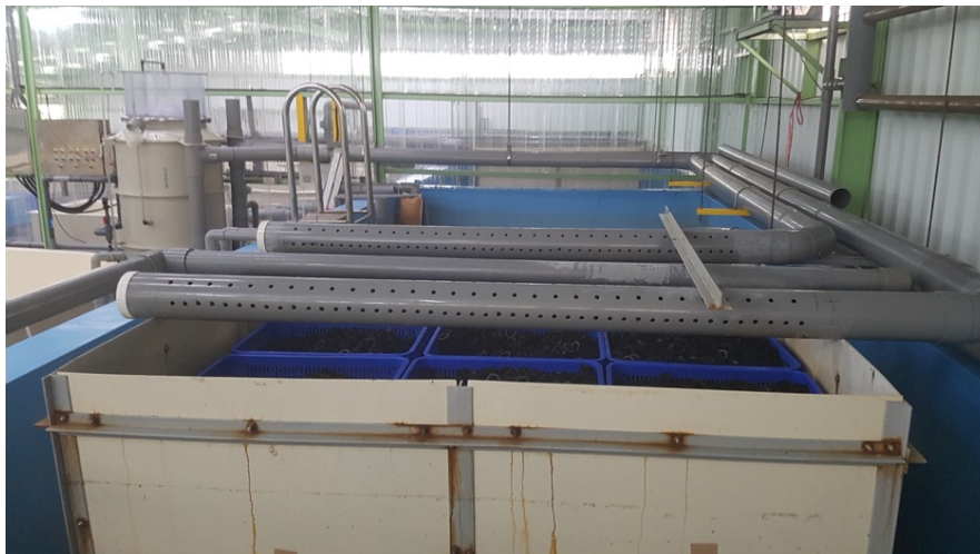
Figure 15: Bio-filter with trickling filter incorporated.
