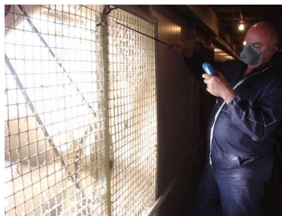
Figure 18: Measurement of airspeed at fan face (Internal)
