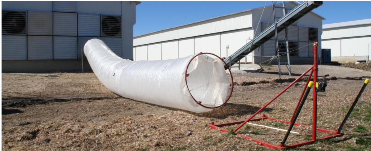
Figure 6: Polyethylene duct attached to tunnel ventilation fan
