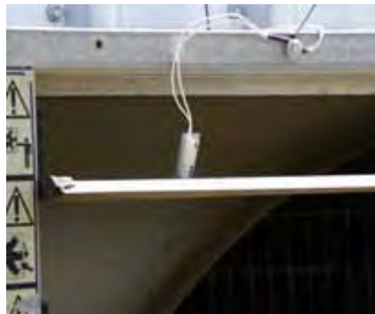
Figure 19: Mercury tilt switch with fan turned on (shutters open, switch open)
