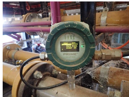
Figure 4. Sage Thermal Mass Flow meter measuring biogas flow to one of the 250 kWe generators.
