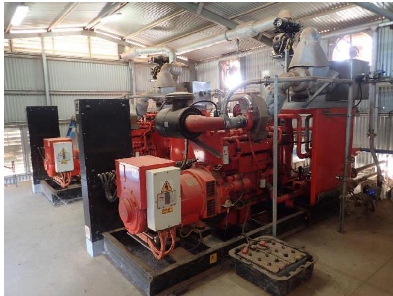
Figure 9. Camda 250 kWe generator units.
