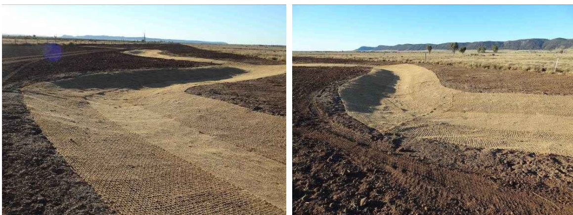
Figure 20. Example of matting along a water course for protection from gully erosion (Fitzroy catchment, Qld).
