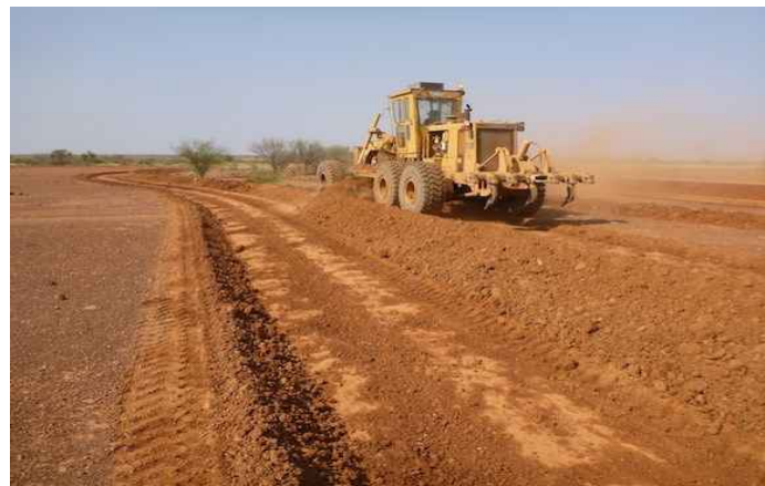
Figure 18. Caterpillar G16 grader building pond banks to a proven design along surveyed contours, Fitzroy catchment, WA. (Photo R. Thompson)
