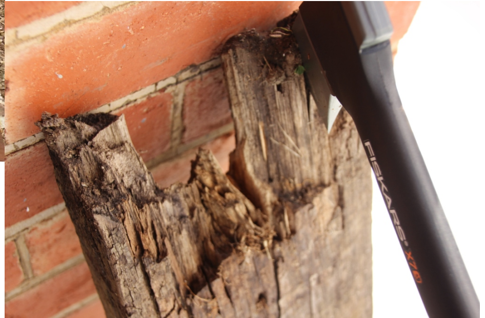
Retaining wall sleeper failure, client: private homeowner
