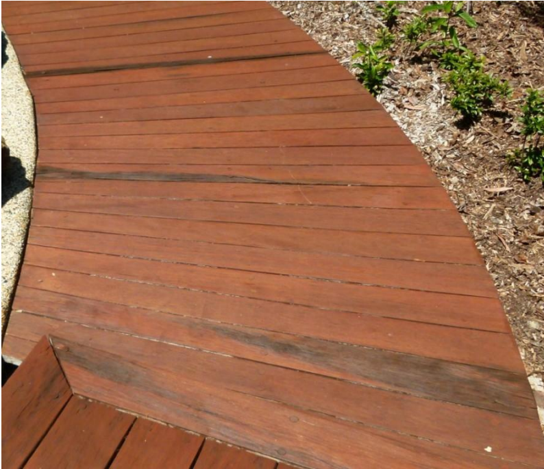
Decking failure, client: private homeowner
