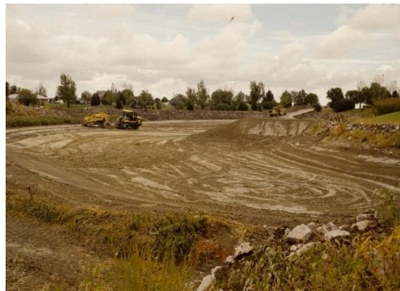
Excavating sediment and re-contouring the substrate topography in a small drained reservoir (image NGP)
