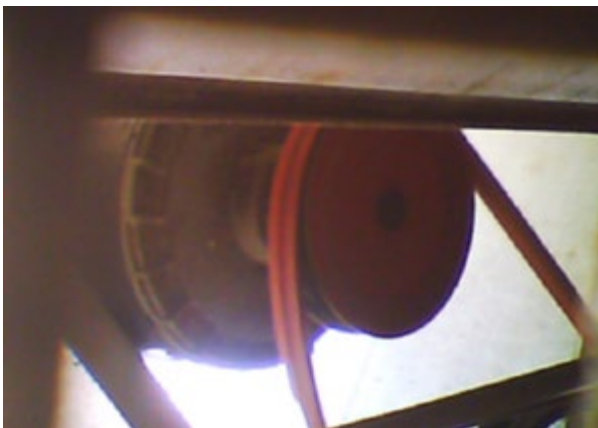
Belt sheave with a loose belt
