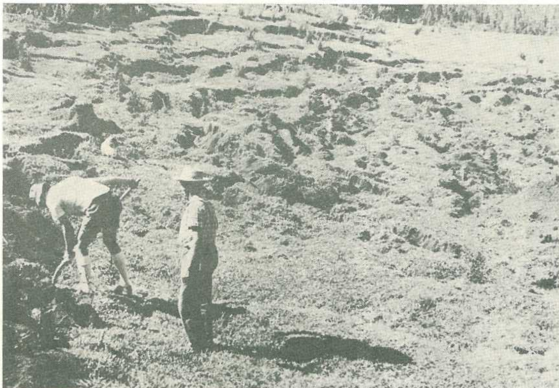
Land slump at Baroon Pocket on kikuyu that was once highly productive. Kudzu ( Pueraria lobata ) has been planted to stabilize the area.
