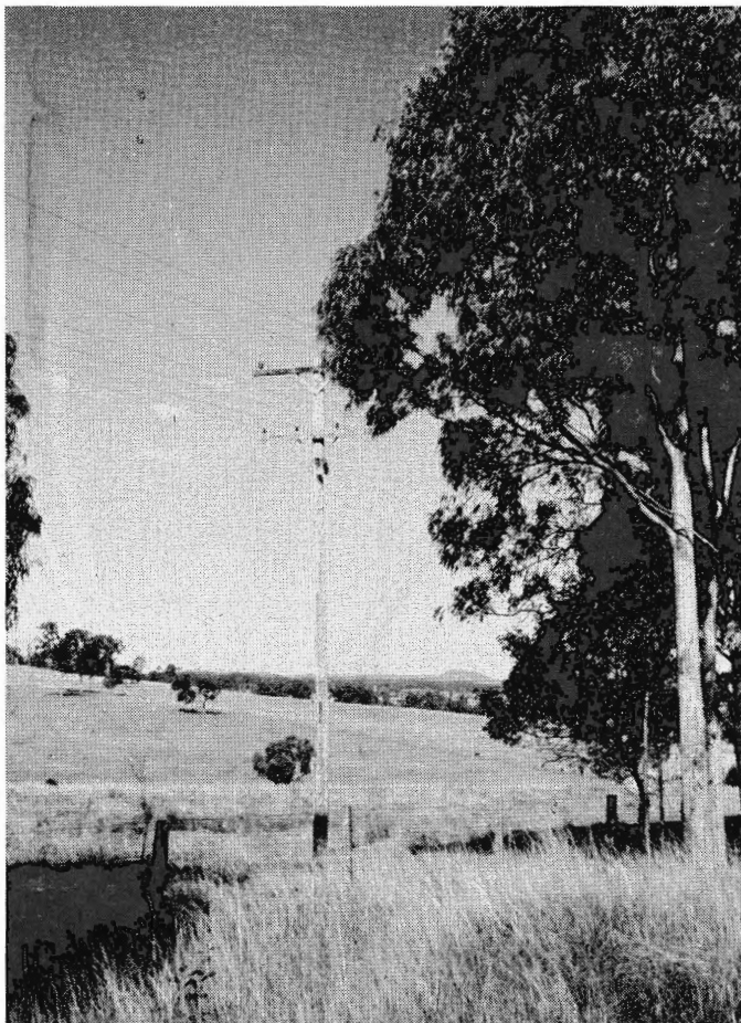
Plate 1. Tall growing trees may interfere with power lines and create a potentially dangerous situation.
